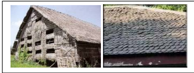
Figure 8 (a). Traditional warehouse in Bantul which is highly resistant to the earthquakes Figure 8 (b). 35 year old roof in Surabaya
