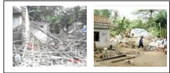
Figure 2. Destruction under Earthquake in Bantul Yogyakarta (May-2006)
